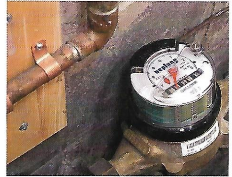
Water meters are the property of the water utility. They should be called if it is leaking or not working properly.
