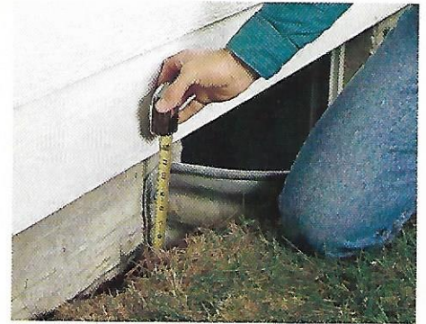
Dripping roofs and leaking gutters can create a gully at the foundation that traps water and fosters leaks.
