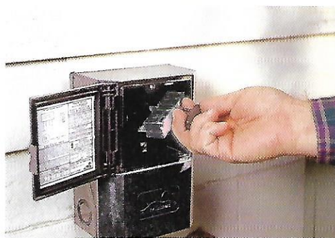
1 The first step is to shut off power to the unit. Most systems have a cutoff box mounted outside near the fan unit.
